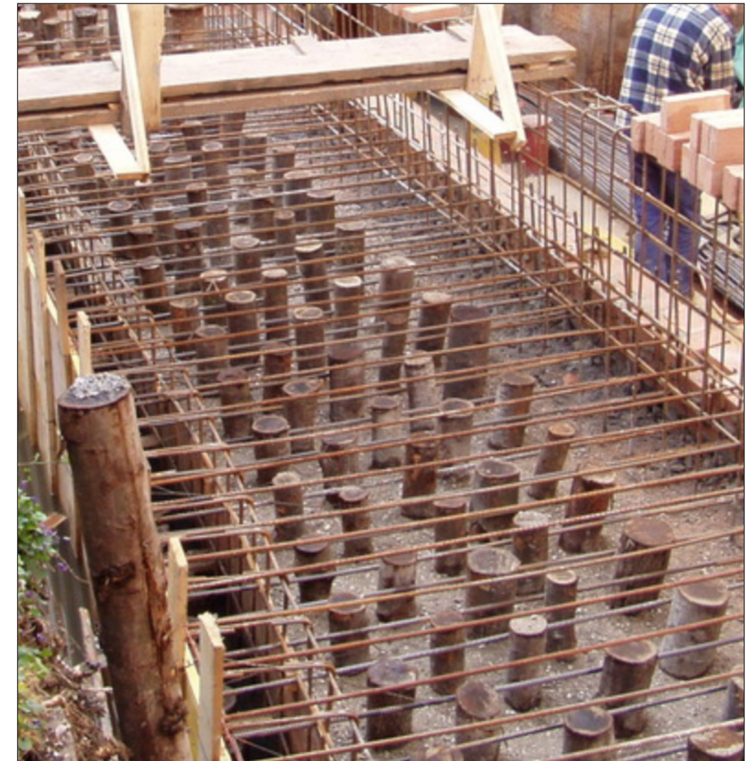
Fig. 20. Excavation and repair of a site in Venice, showing foundation pilings. Allo Squero, Venice, It.
