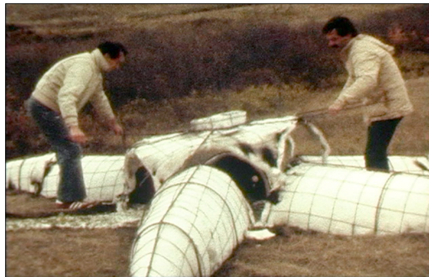
Fig. 55-57. Construction, installation and post-fire dismantling of the kiln. Video stills from John Roloff, A Project for Regina, an Outdoor Firing , produced by the Norman Mackenzie Art Gallery, September, 1980.
