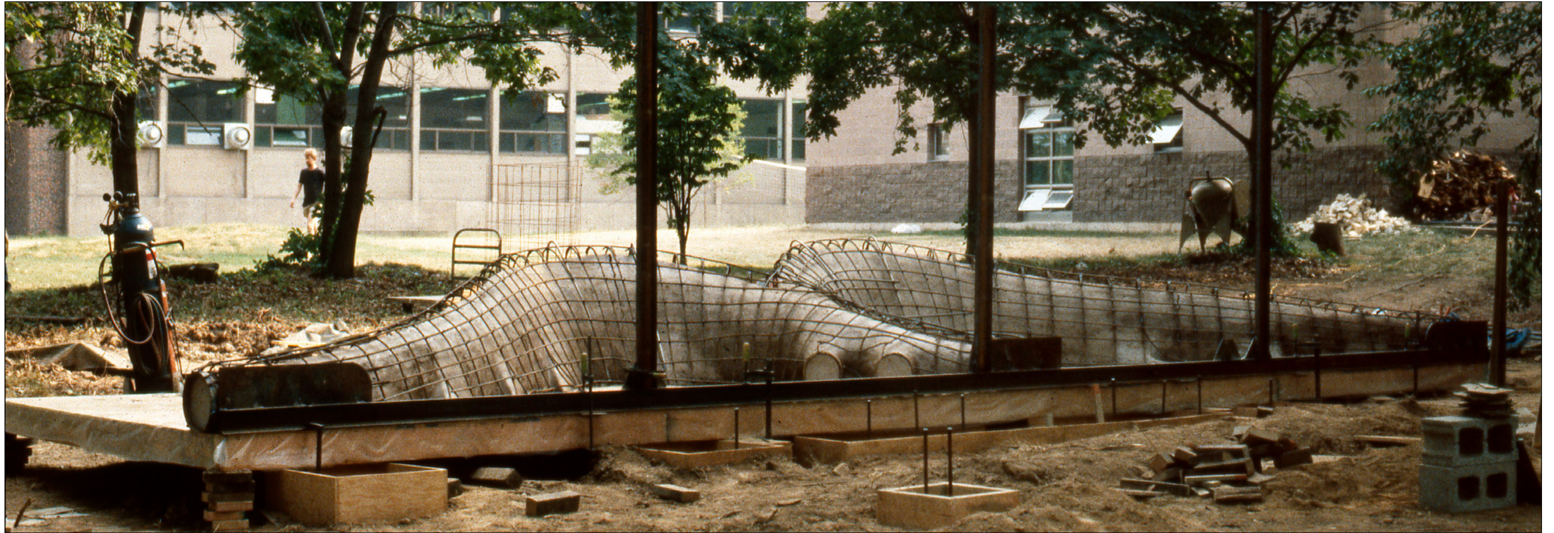
Fig. 153. Untitled (Earth Orchid) , mold core with rebar/pre-refractory cement placement/horizontal position, 32 ft. l., steel, clay, wood, concrete, 1988.
