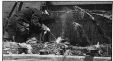
Above, Mort Scott welds rebar during the initial stages of sculpture construction.
