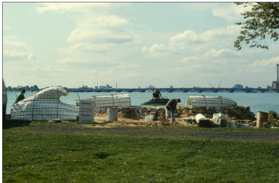
Fig. 112. Wave Ship (of Fire) , installation, glass ship element, Owen Park, Detroit, MI, 1984.
