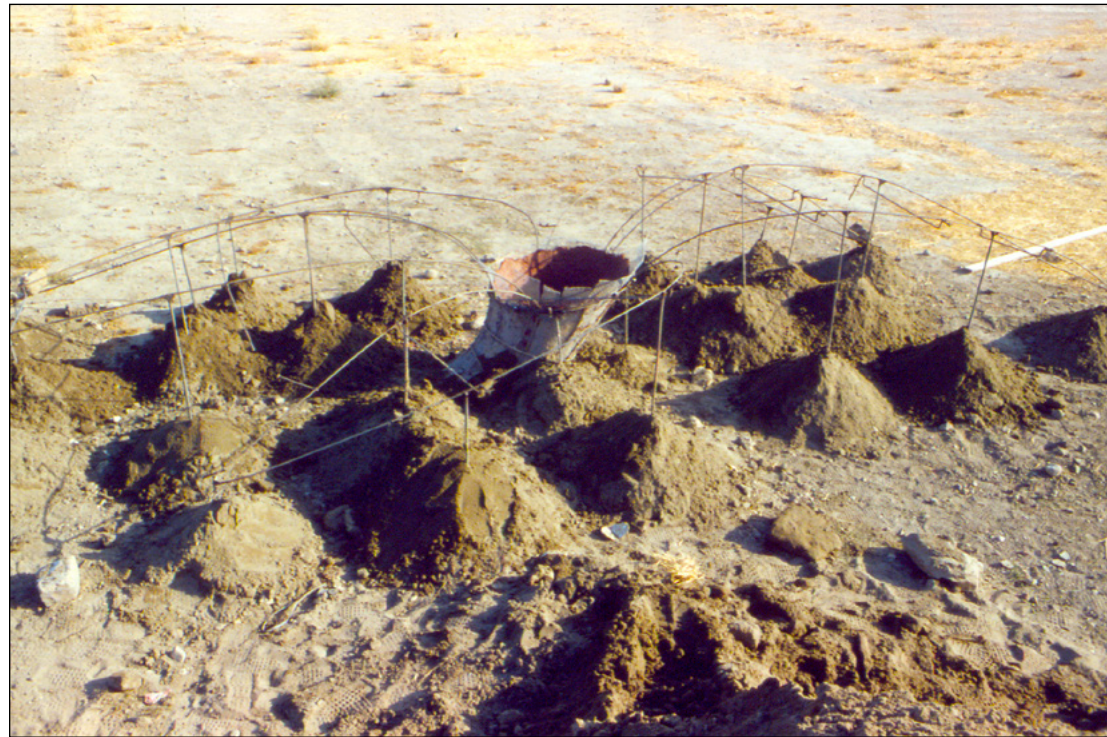
Fig. 86. Mountain Kiln/Black Orchid , installation of metal armature for the kiln's orchid floor, the central orchid's 'throat' connected underground to a sheet metal flue off-camera to left of image and armature where sand will be brought up to the orchid's petal surface.
